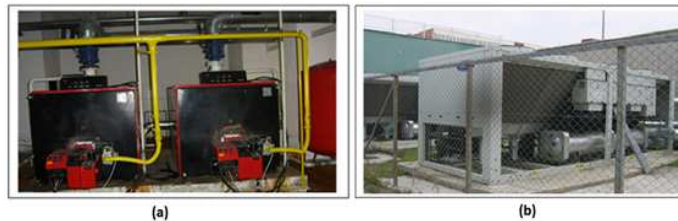
FIGURE 3. In the example building, a) Heating system boiler, b) Cooling system (chiller).
