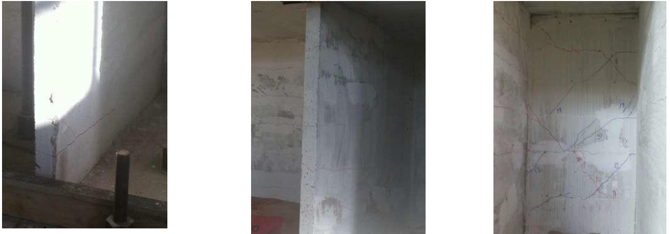
Fig. 10. Crack patterns on the existing tunnel form building model before collapse.
