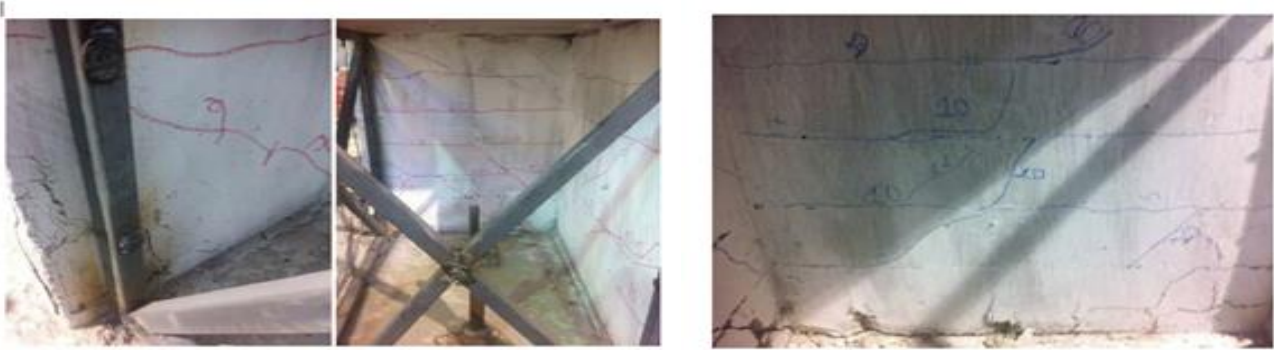
(b) Cracks on first-story shear walls
