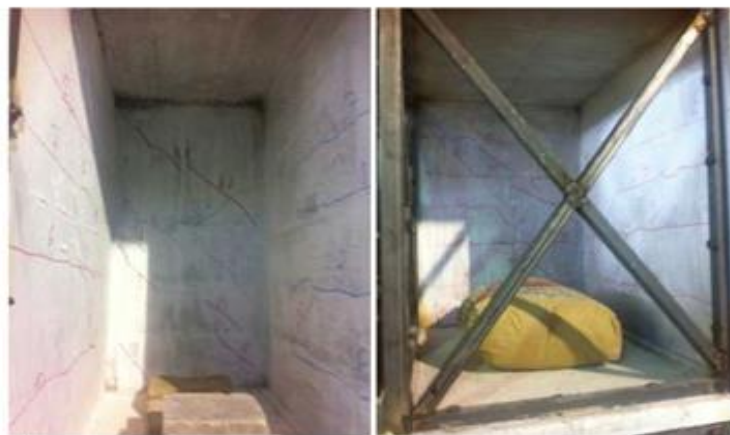
(a) Cracks on second-story shear walls
