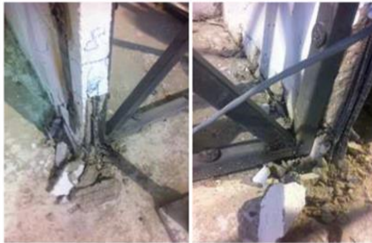
(c) Damage at wall and steel brace connections at the foundation level
