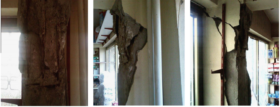
Fig. 2. Damage pattern in the column in which shear hinge was observed.
