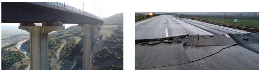
Fig. 35 Viaduct on TAG Highway: no damage to deck, columns, or supports; Tarsus-Adana-Gaziantep Highway: observed damage
