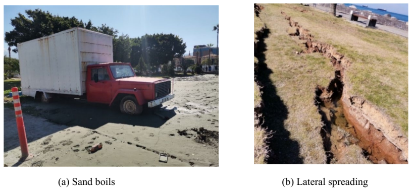
Fig. 18 Liquefaction-induced ground deformations in Iskenderun/ Hatay
