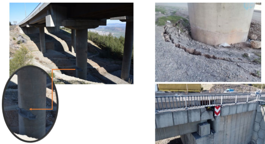
Fig. 36 Damage observations on TAG highway viaduct
