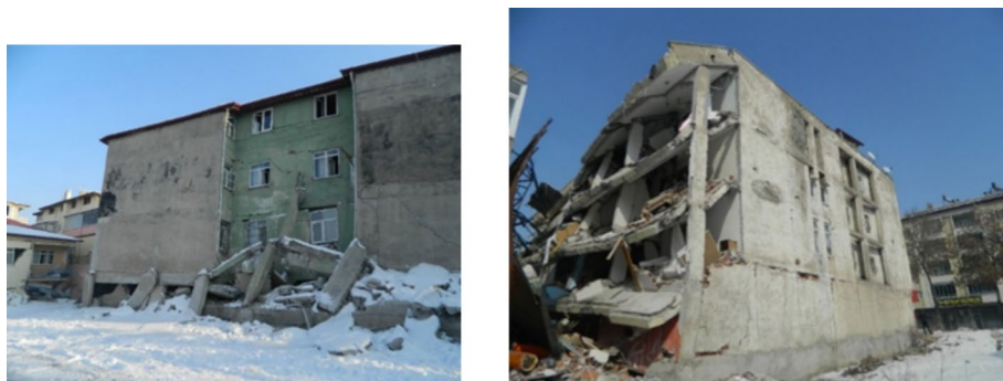
Fig. 24 Partially collapsed buildings
