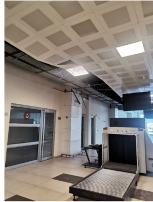
(b) Main building suspended ceiling damage
