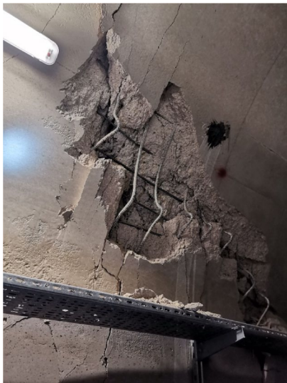
(b) Partial damage to the tunnel
