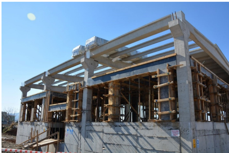
Fig. 27 Structural damages (buckling in column reinforcements) in a new construction in a textile facility in Kahramanmaraş
