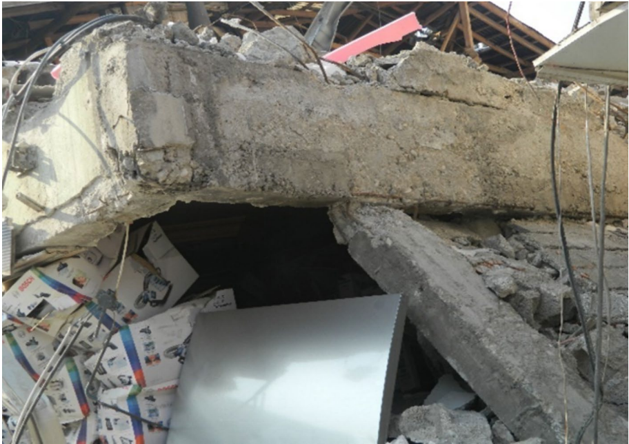
Fig. 22 Observed design problem as strong beam-weak column
