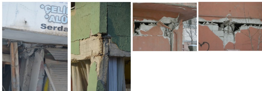
Fig. 21 Problems observed with insufficient beam-column joint details
