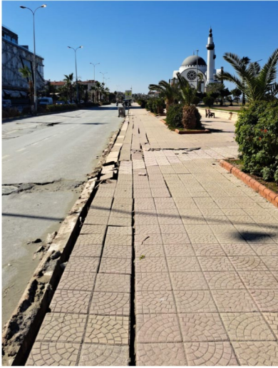
(a) Damages on the road and pavement due to liquefaction in Iskenderun
