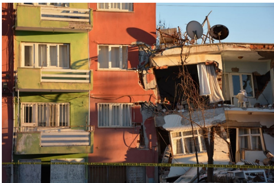
Fig. 25 Pounding effect observed in adjacent buildings
