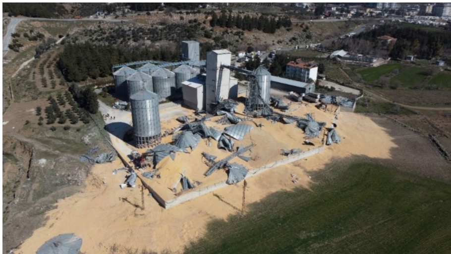
Fig. 29 A food facility in Gaziantep Nurdagi with damaged corn and wheat silos
