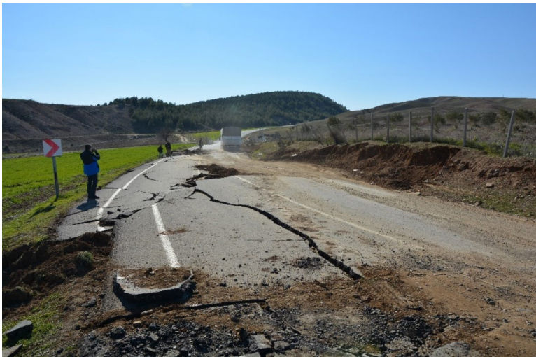
Fig. 39 Damage observations at Pazarcik—Tevekkeli village road and fault intersection
