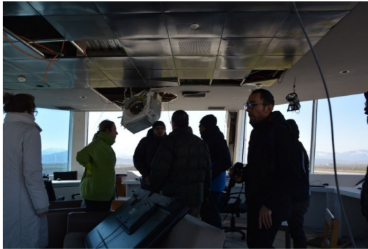
(a) Non-structural damage to the tower structure
