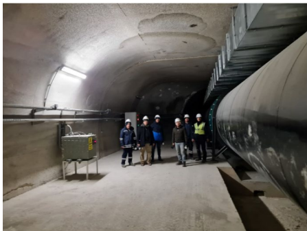
(a) Duzbag drinking water transmission line and tunnel
