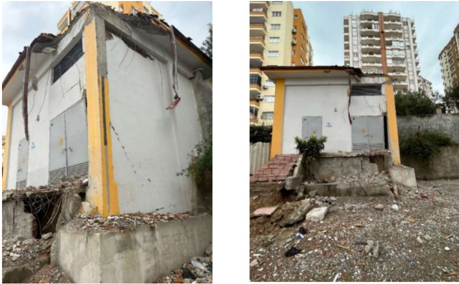
Fig. 34 Adana City Transformer Center TR184 Damage (Toprak et al. 2024b)
