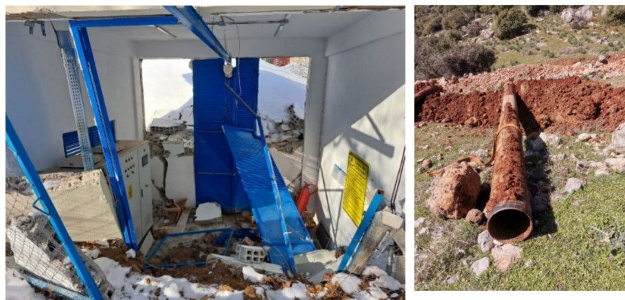
Fig. 31 Damages in water systems caused by fault movement
