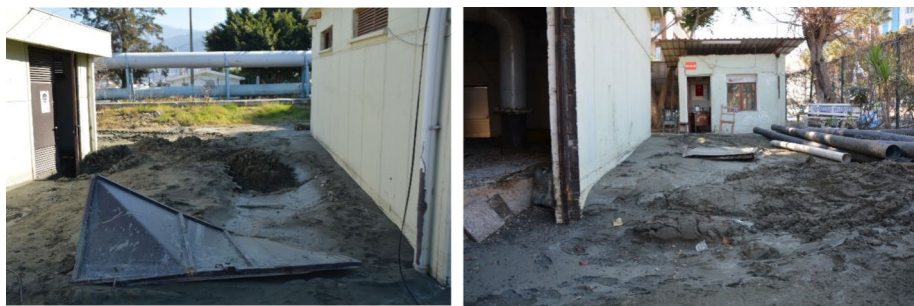
Fig. 32 Damages caused by liquefaction at the sewerage and storm water elevation station in Iskenderun
