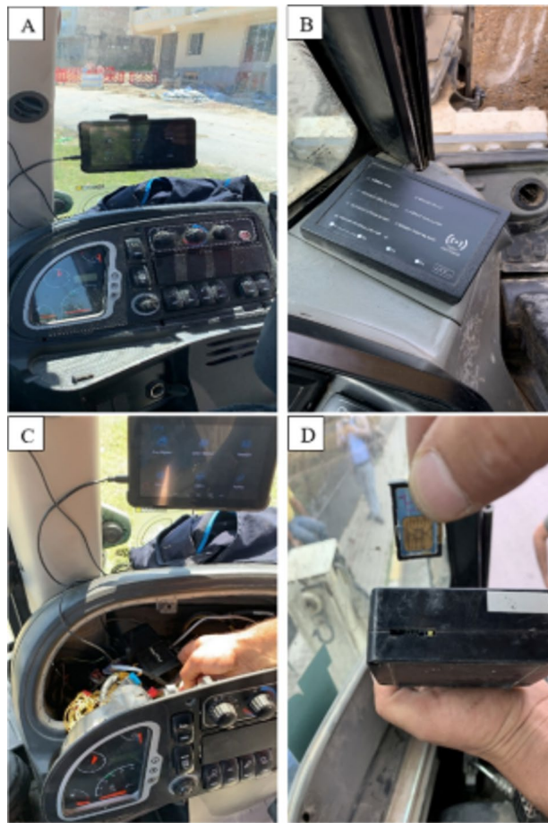
Fig. 4. Onboard hardware configuration of the excavation tracking unit (a) in-cab operator display, (b) RFID-based authorization reader, (c) onboard control unit, (d) cellular communication module.
