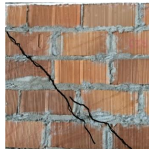
Fig. 4 Damages of the cement mortar walls
