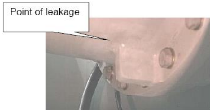
Figure 3. Point of SF6 gas leakage
