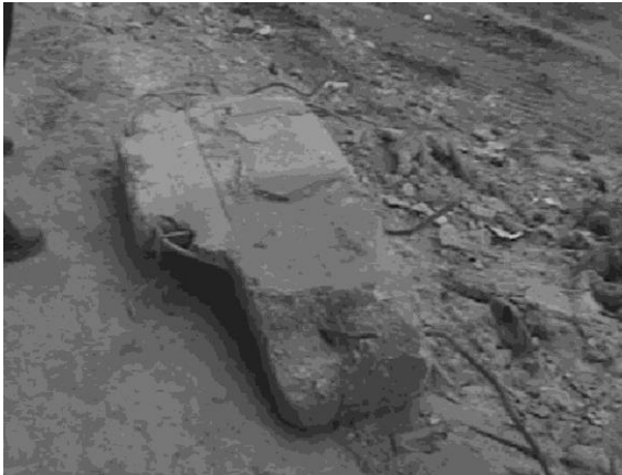
Fig. 10. Column found in debris with variable cross-section (Bottom part 25/40 cm, upper part 25/70cm) at the ground level.
