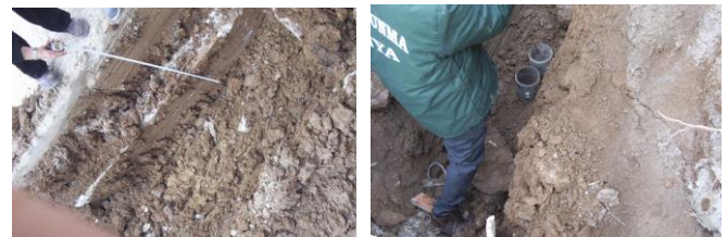
Fig. 9. Soil samples and foundation depth.
