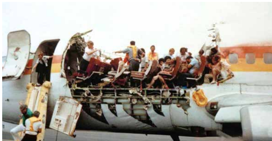
Figure 1. The 1988 Aloha Airlines Incident Occurred due to Lap-Joint of Fuselage Fatigue Failure
