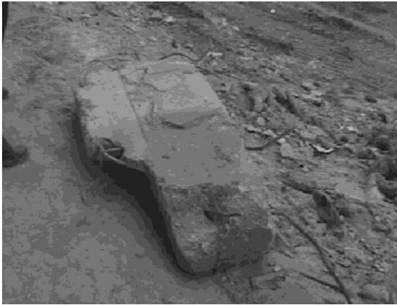
Fig. 10. Column found in debris with variable cross-section (Bottom part 25/40 cm, upper part 25/70cm) at the ground level.
