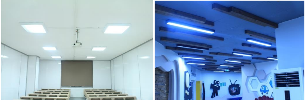
Picture 1. Some areas where A, B and C Block lighting works are carried out
