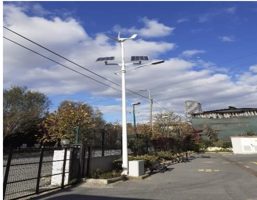
Picture 5. D block solar and wind powered environmental lighting pole
